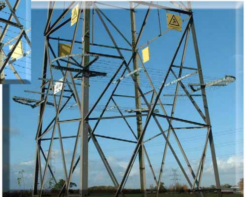
132kV TOWER ACD's
