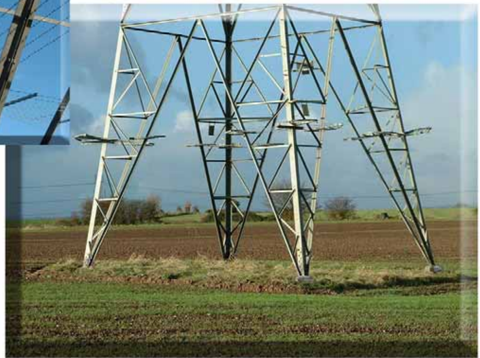
275kV AND 400kV NGC TOWER ACD's
